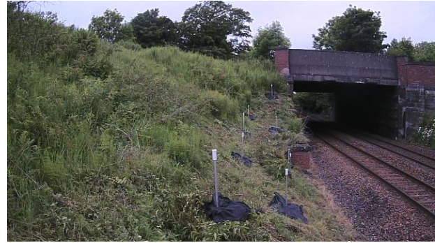
130k+ embankment monitoring in UK
