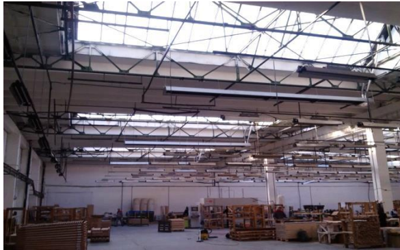
Industry hall heating
